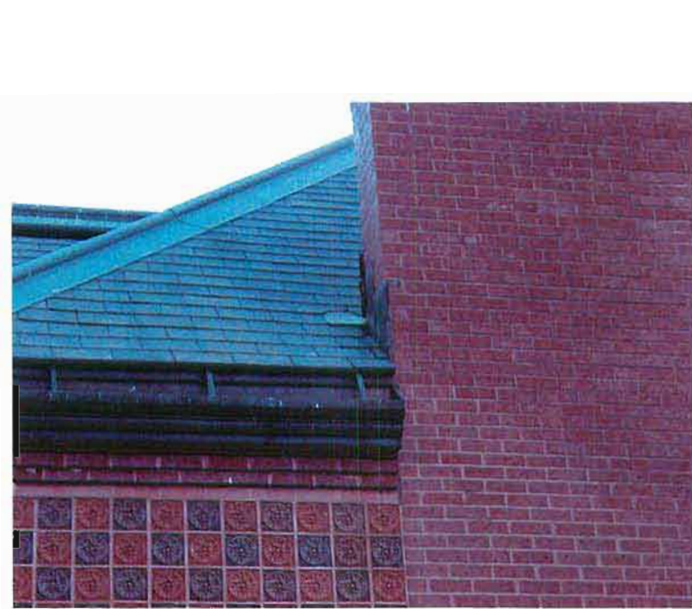
Corner at LL and Bedford – broken tile
