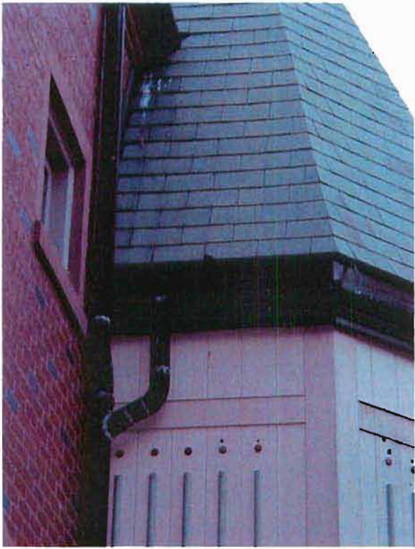
First floor turret facing Trapelo Road - broken tile
