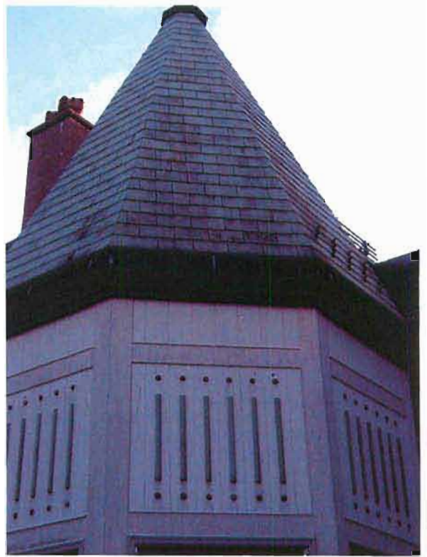
First floor turret facing LL and terrace – worn tiles
