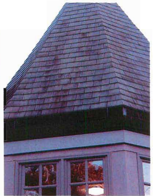
Story room turret – worn tiles
